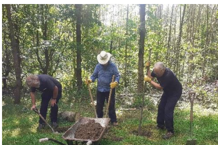
Digging the holes for the uprights of the bench on the main ride.
